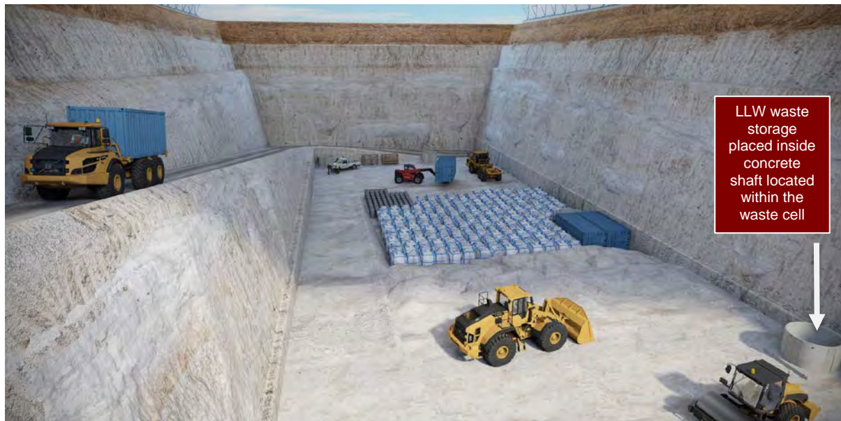
Figure 5-21 Radioactive waste storage (shaft in cell)
